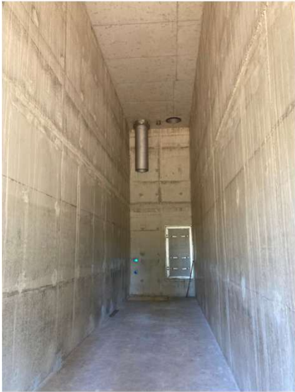
Inside the ozone contact tank
